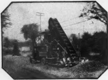
At Stockpile, Batching Aggregates for Paving Mixer. For this work, Hais loaders are equipped with the Precision Strike-off Measuring Hopper.
